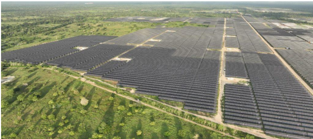
Bild 2 Guayepo I & II Solar Park. Credit: Enel Green Power 6
